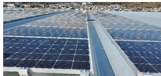
Solar power panels installed on the roof
