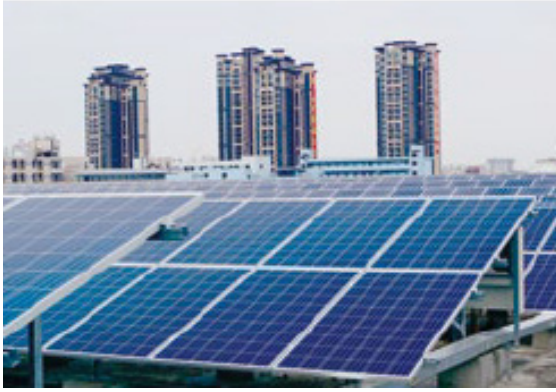
Solar power panels installed on the roof Left: Konica Minolta Business Technologies (Dongguan) Co., Ltd.
